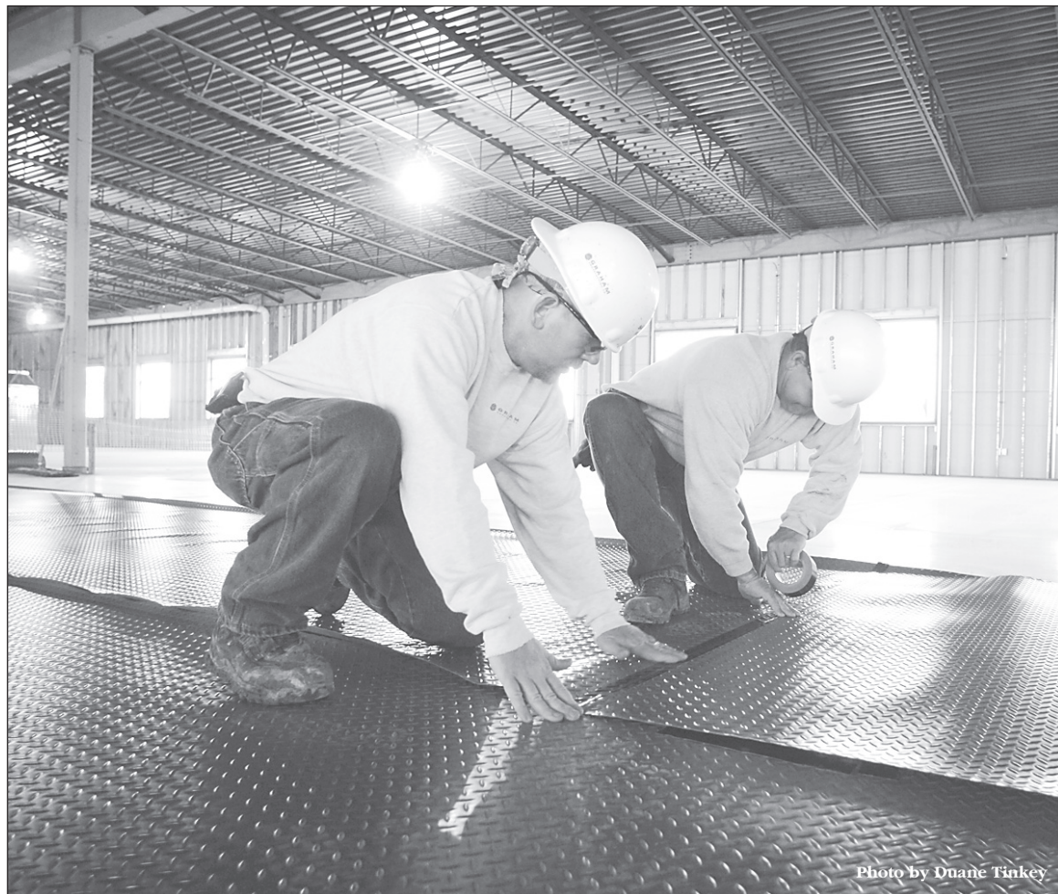
Mike Sullivan, left, and Henry Norman of Graham Construction Co. secure a protective cover to a newly polished concrete floor at a building under construction in Ankeny.
